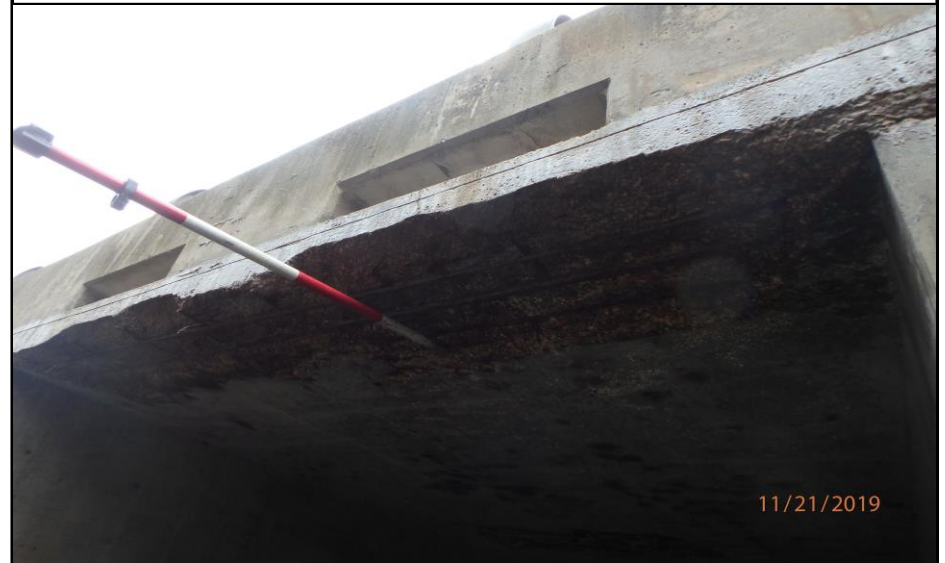
2.5ft. Spall and Exposed Rebar, South End of All Cells - Looking North
