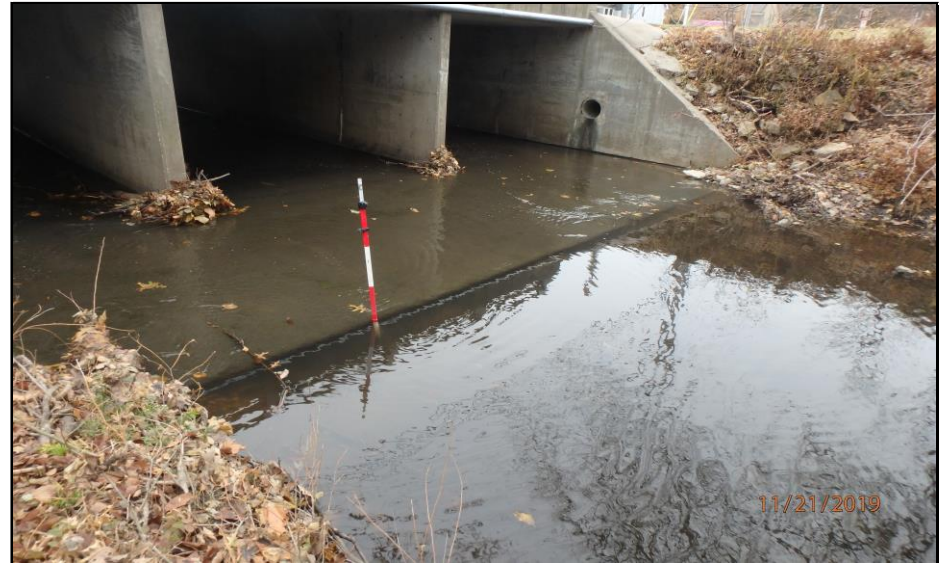
1 ft. of Scour Full Width of Upstream Toewall - Looking Southwest
