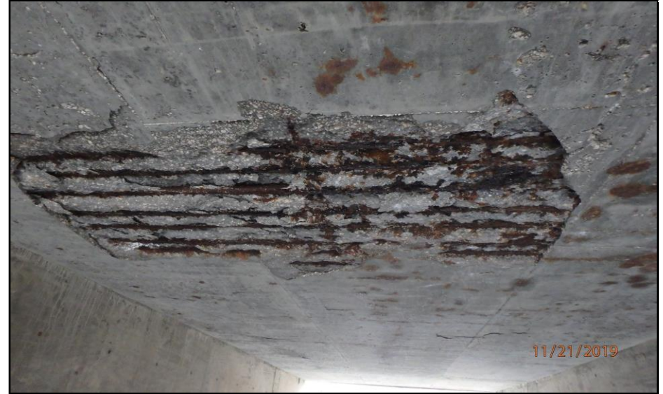
3 ft. by 8 ft. Spall with Exposed Rebar in Ceiling of Center Cell - Looking North
