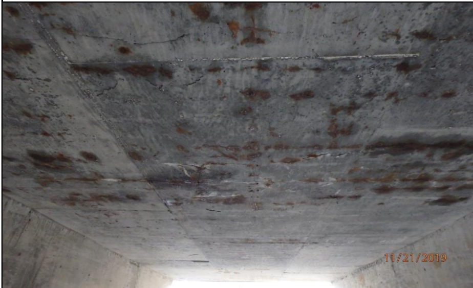
Typical Ceiling Deterioration in East Cell - Looking North
