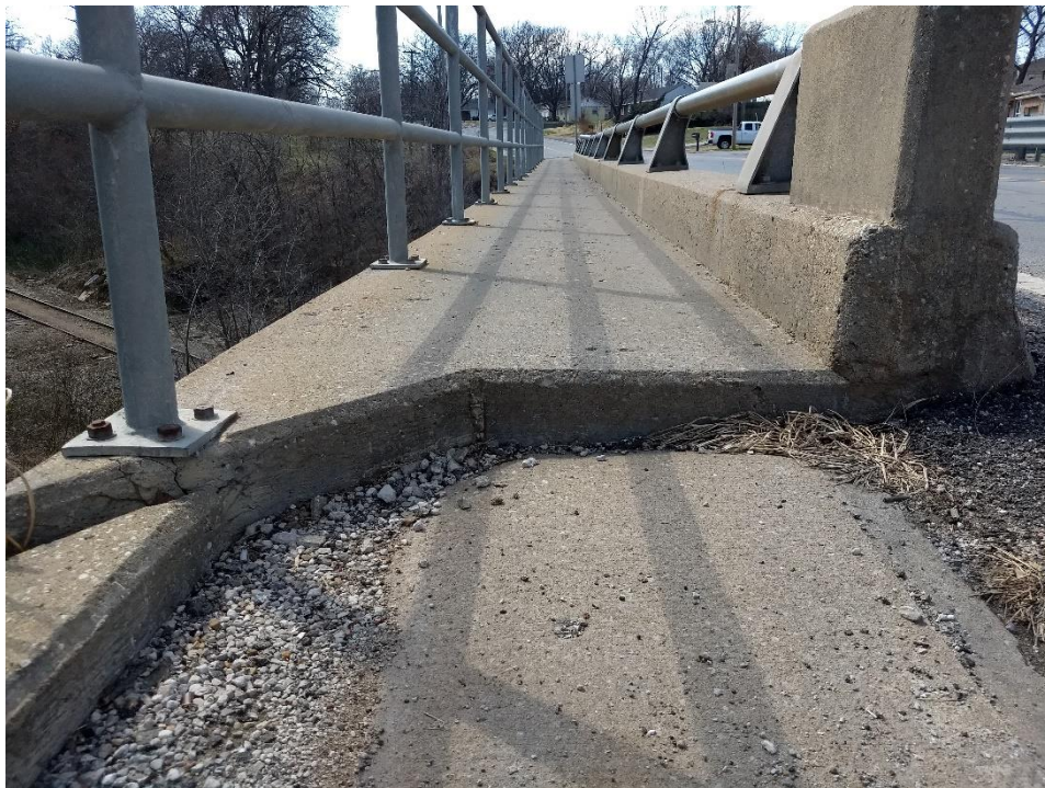
83 rd Street looking west. Steps at either end of sidewalk on bridge discourage the use of the sidewalk and prevents wheelchair access.
