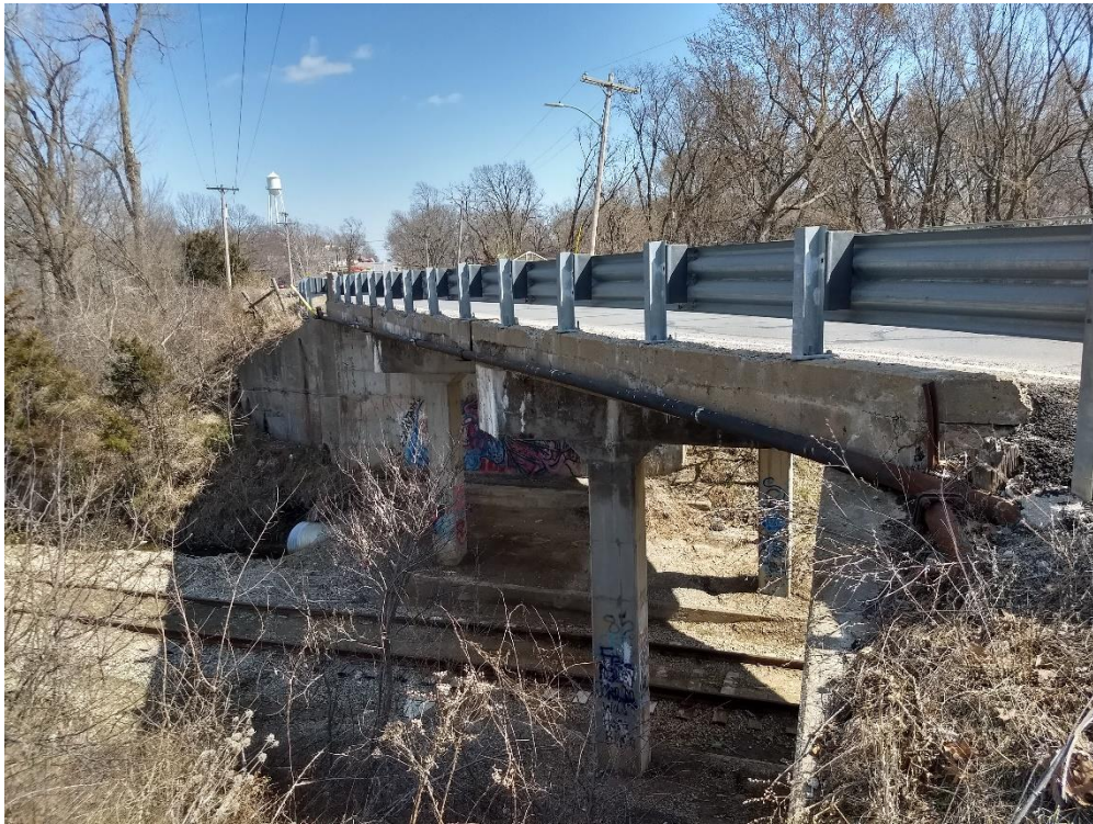
View of the north bridge fascia. Concrete under 2007 guardrail retrofit continue to deteriorate and loose concrete anchorage.
