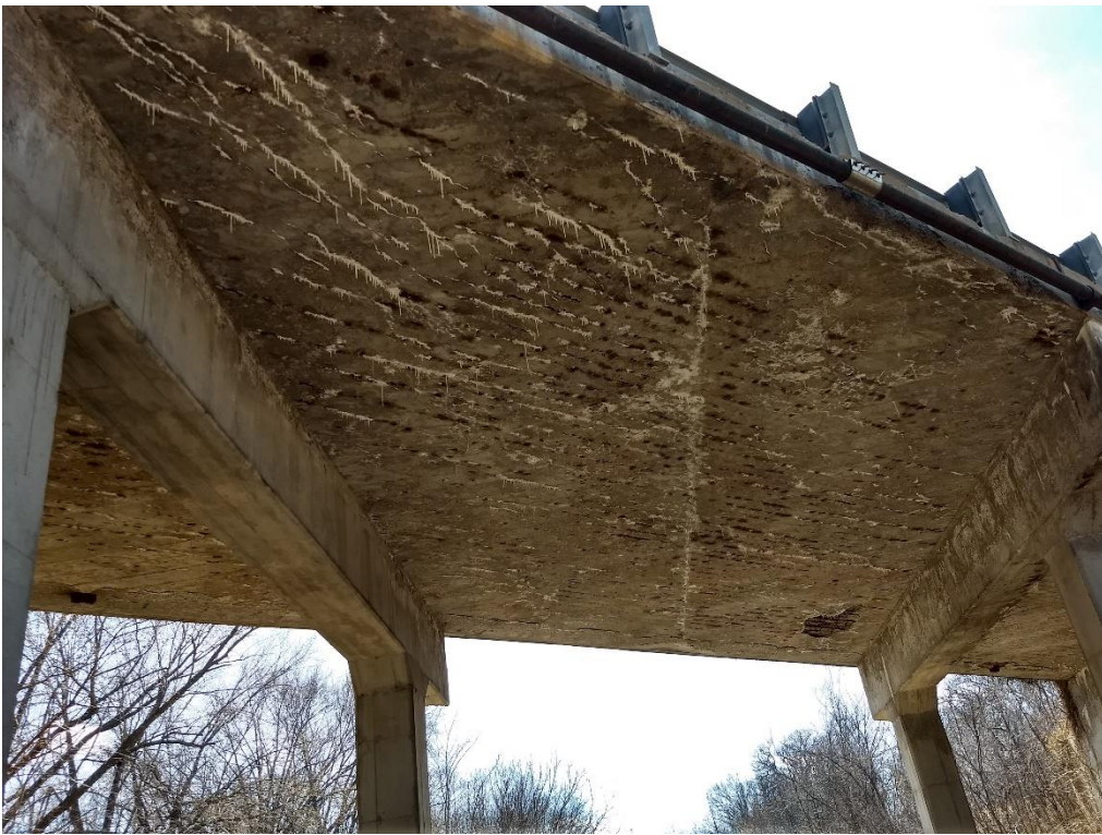
View of underside of bridge deck. Continued deterioration if not repaired or replaced will cause the load rating to decrease potentially preventing Emergency Services from using bridge.
