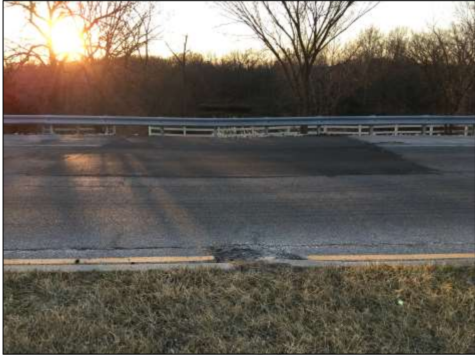
Figure 2 – Photograph of Northbound Raytown Road Pavement Sagging on Top of Existing CMP Source: WSP (March 15, 2018)
