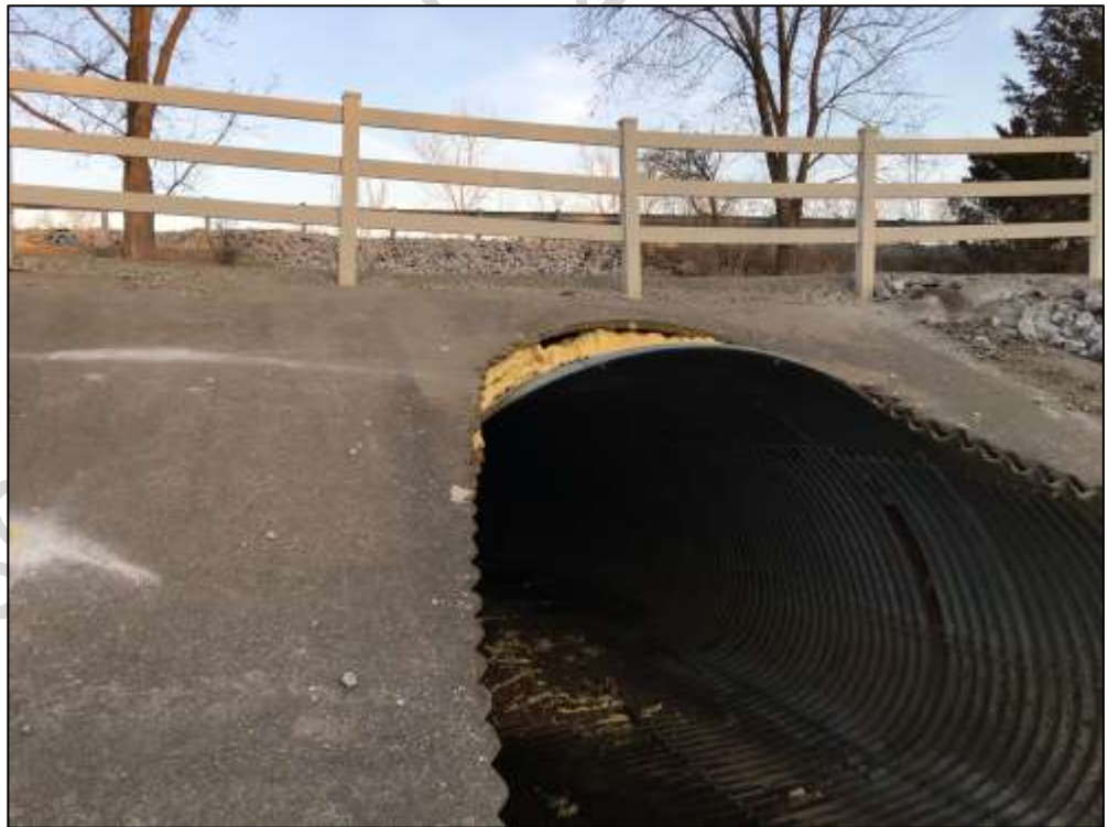
Figure 1– Photograph of Existing CMP (1 of 2 CMPs) under Northbound Raytown Road Source: WSP, March 15, 2018
