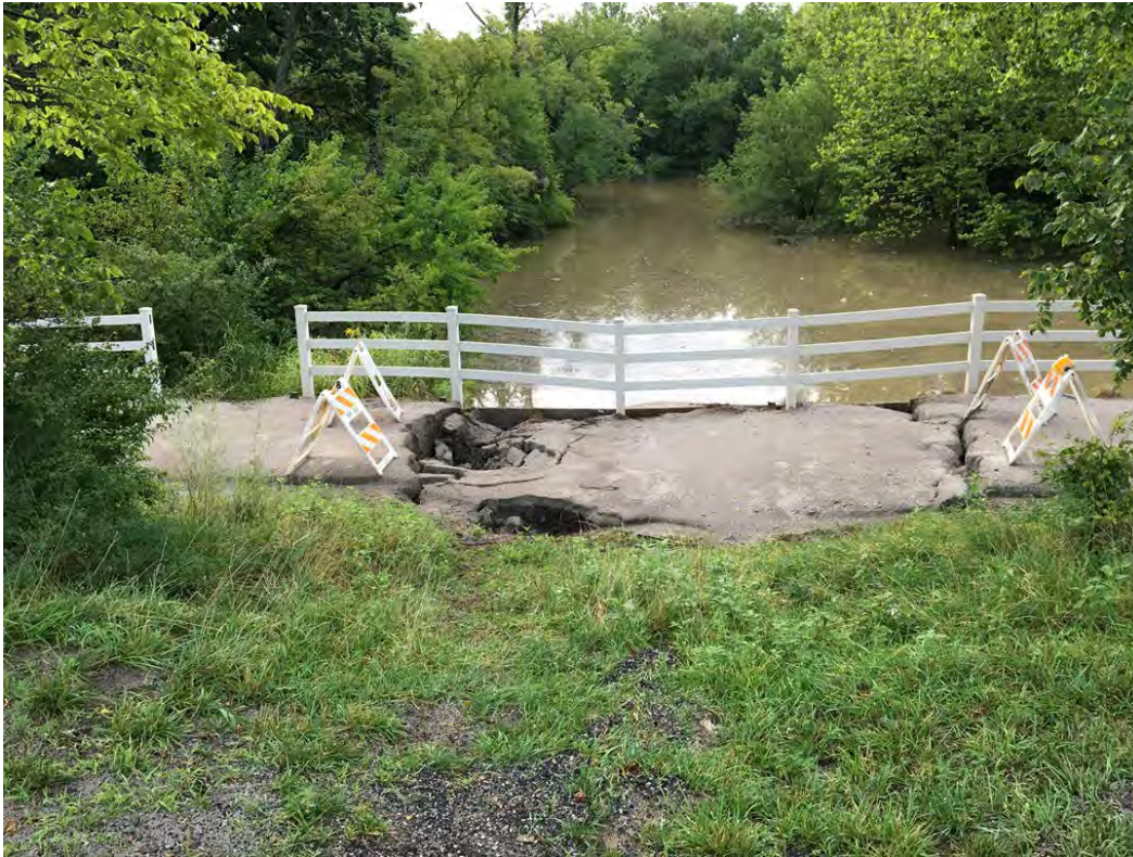
Photo 1 – looking east at the failed portion of the shared-use trail from Raytown Rd, 8-6-2017.
