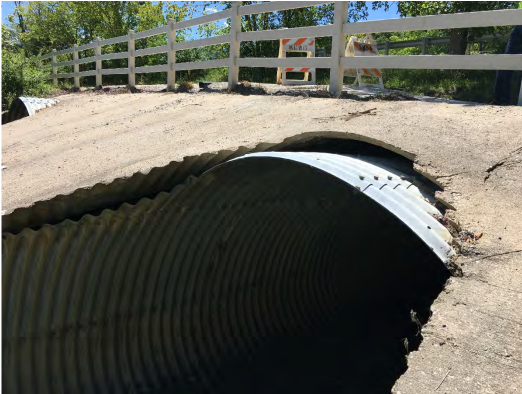
Photo 9 – downstream end of the north culvert showing 8" gap between the concrete apron and the top of the culvert.
