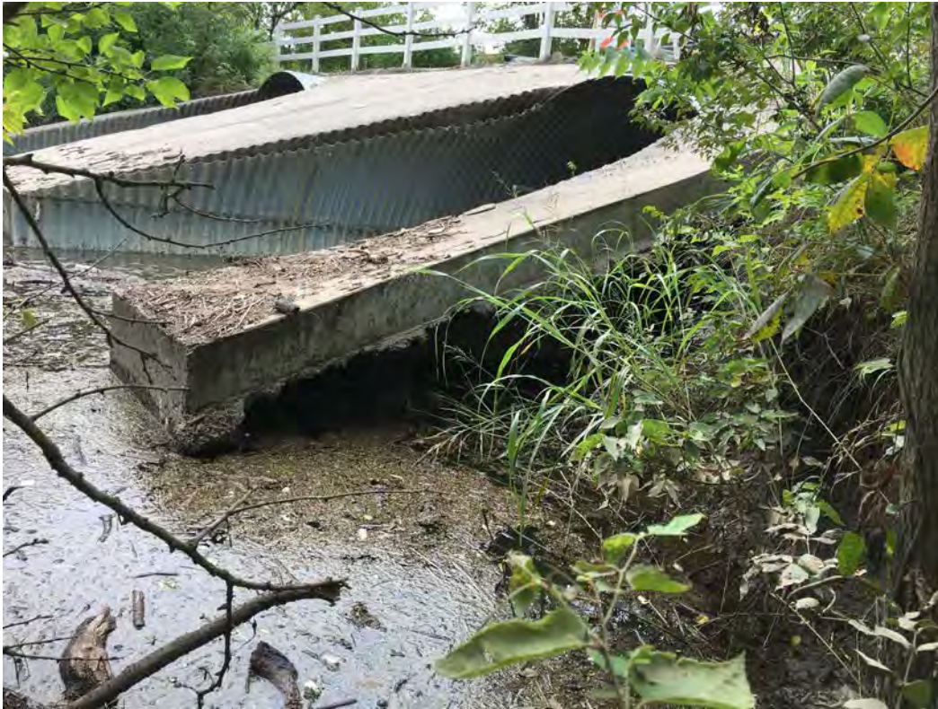
Photo 3 – looking south towards the exposed outside face at the downstream end of the north culvert.
