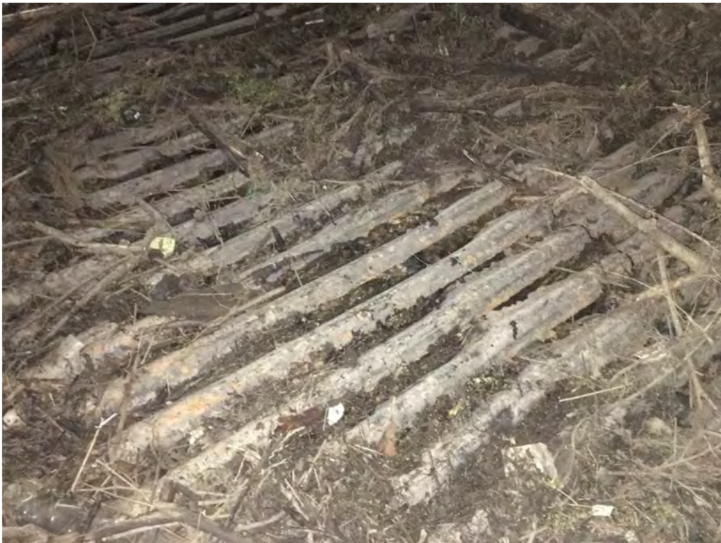
Photo 8 – general condition of the bottom corrugations in the north culvert.
