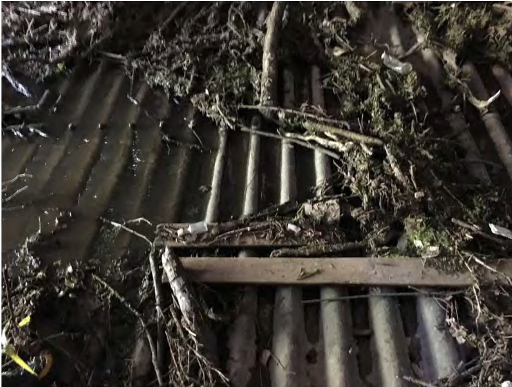
Photo 7 – water running thru the deteriorated corrugations of the north culvert at roughly 40' from the upstream end.
