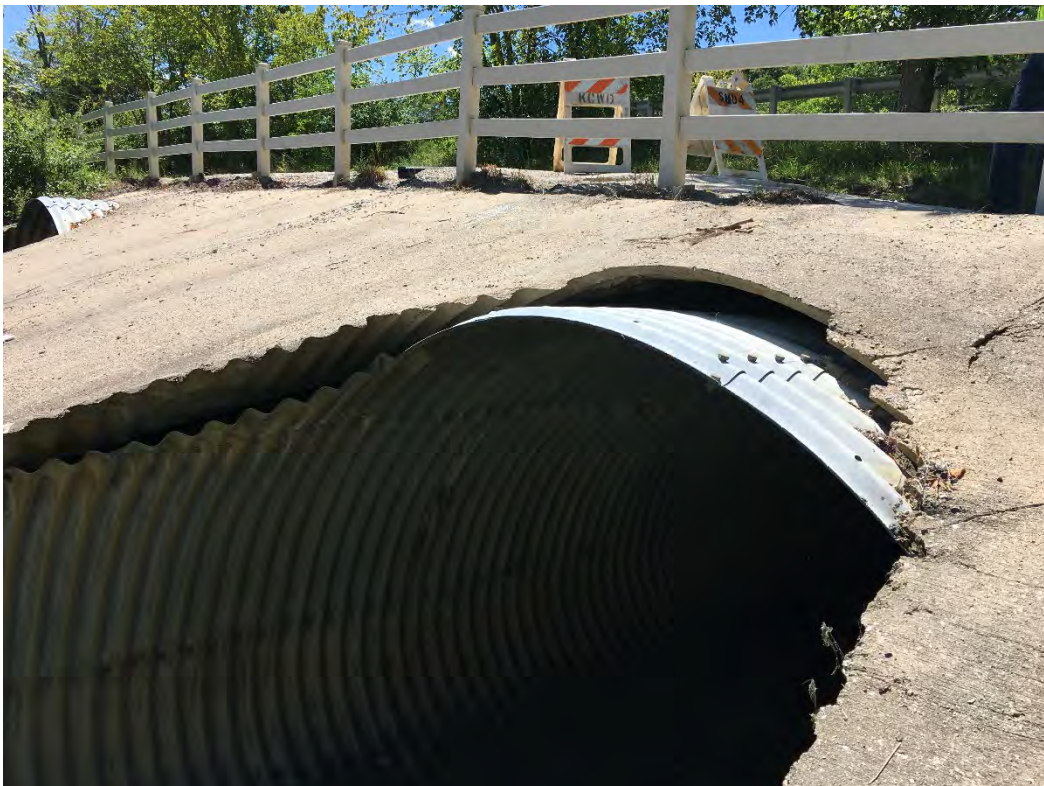
Photo 4 – downstream end of the north culvert showing 8" gap between the concrete apron and the top of the culvert.
