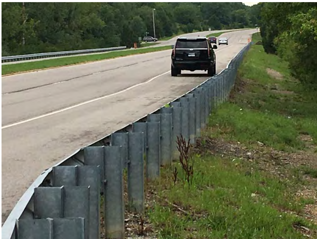
Photo 12 – depression in the northbound shoulder and right lane of Raytown Road.
